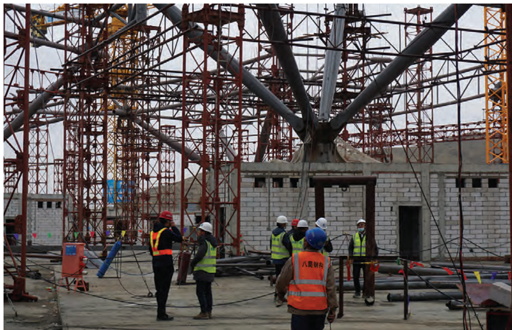
TOP AND ABOVE: Arup also developed an innovative dual directional spherical bearing connection to reduce the member dimensions of the tree columns under the high temperature variation of Lhasa, retaining the architectural intent of a light and elegant roof.
