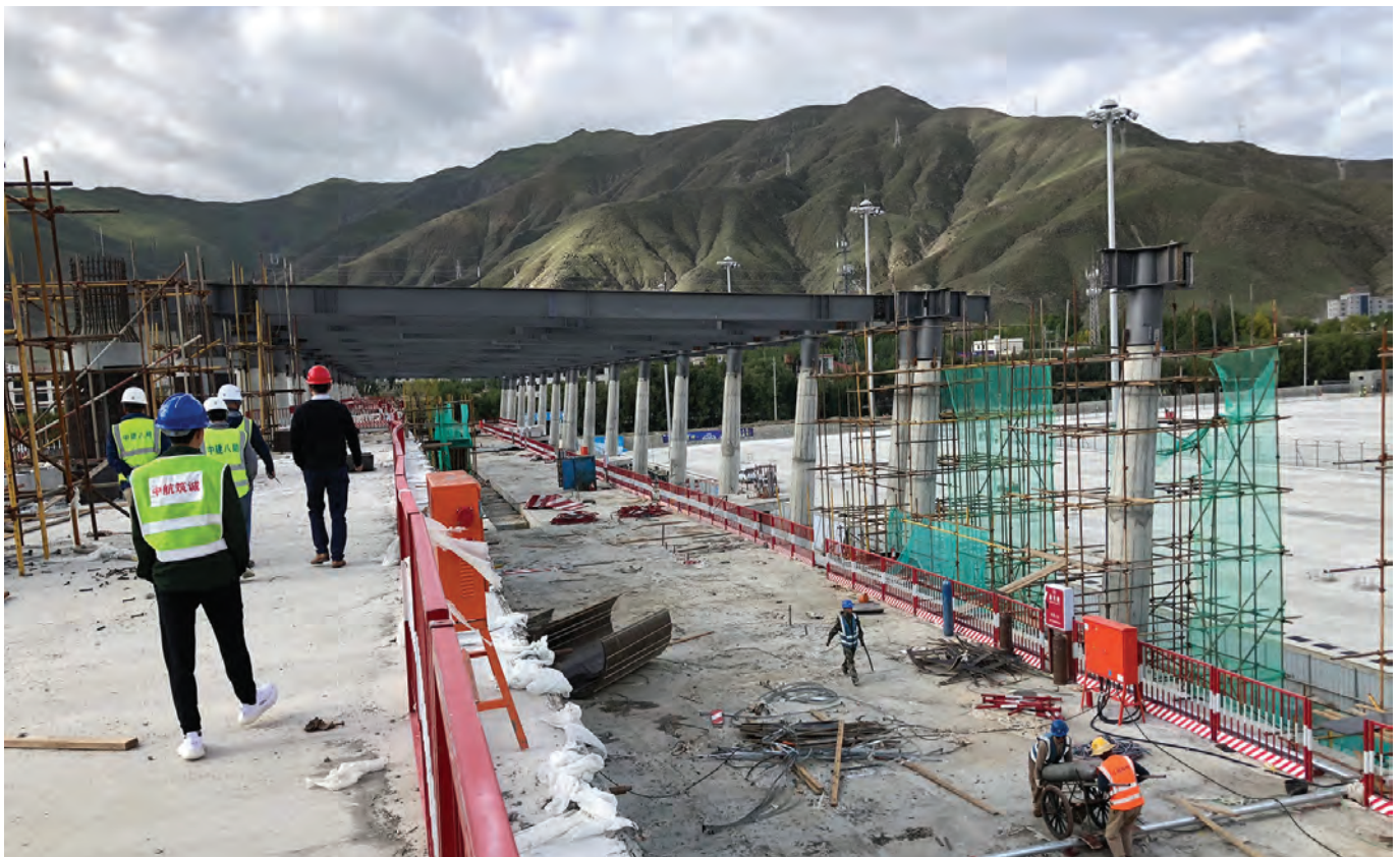
TOP AND ABOVE: Featuring a lotus-shaped roof, the design of Lhasa Gonggar Airport Terminal 3 pays homage to Tibetan culture and ethnic identity. Arup provided a full stage structural, mechanical, electrical and public health engineering (SMEP) design for the new terminal, and technical review for the ancillary buildings.
